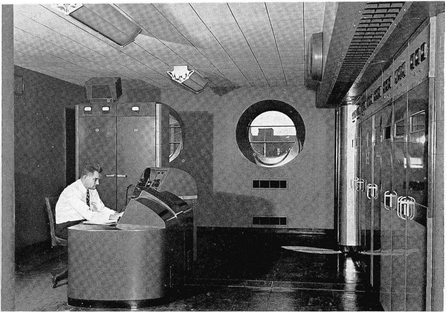
FIG. 6 (above). Transmitter Room view showing flush mounted RCA transmitter, Supervisory Control Console and equipment racks. Mr. Gordon Rustemeyer, Transmitter Supervisor, is shown at the controls.
