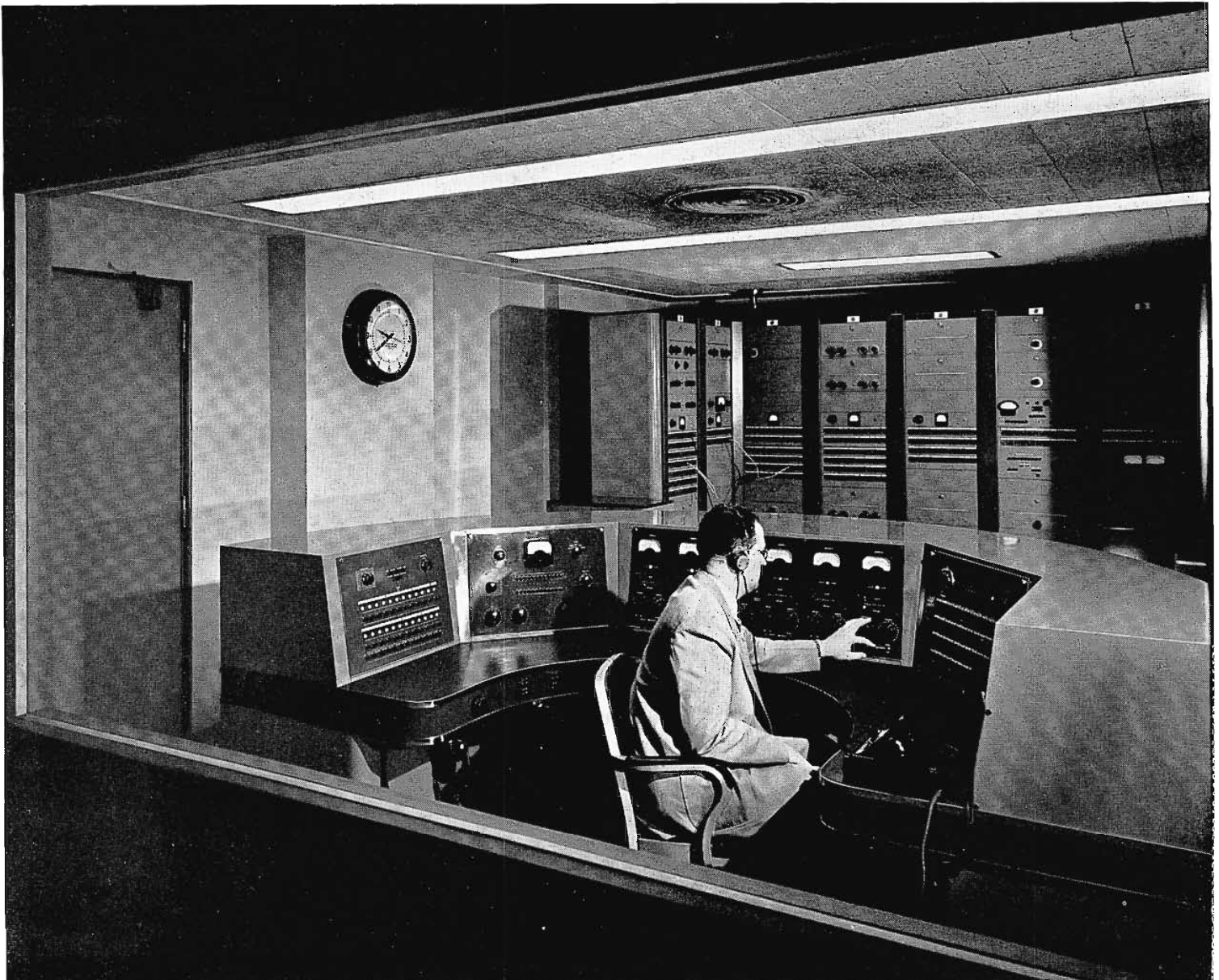
FIG. 1 (below). View of the Master Control Room at the new KSD Studios showing the control console in front and nine Deluxe Audio Equipment Racks at the rear. All AM program control functions are handled from this point.
